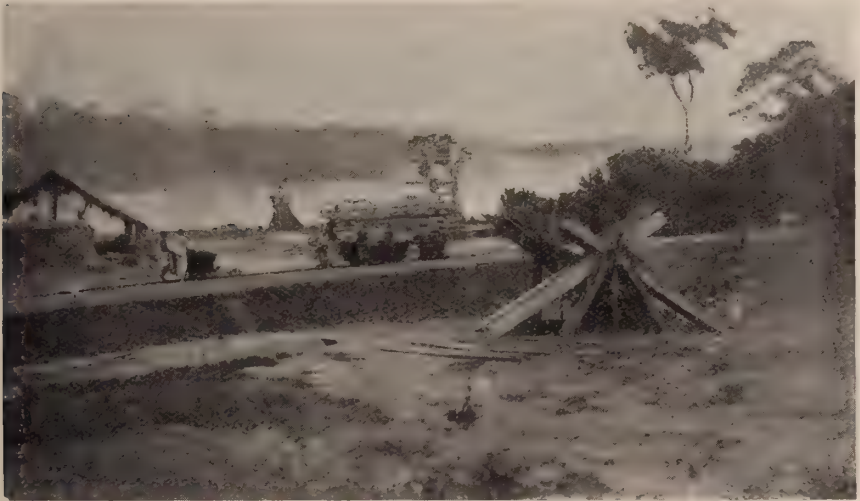
165. THE RAILWAY LINE ALONG THE LUALABA-CONGO NEAR PONTHERVILLE, OPPOSITE THE MOUTH OF THE LILU RIVER
